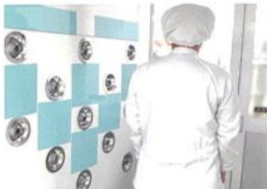
On the wall in air shower
